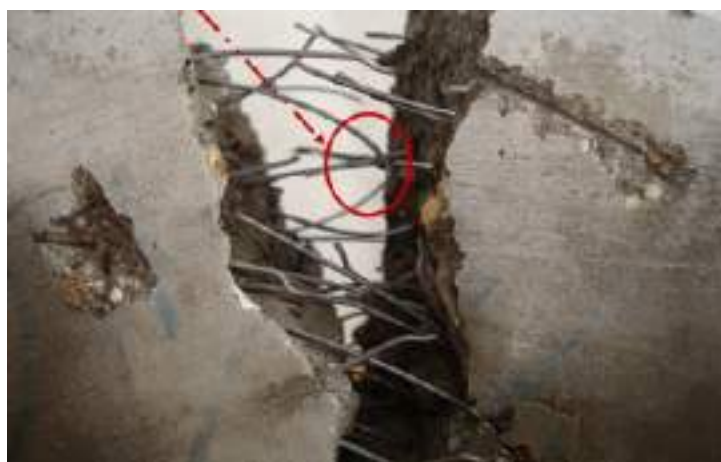
Figure 9. Prevention of Cracks (bringing by fibers) [39] Used as per Elesivior Permissions.
