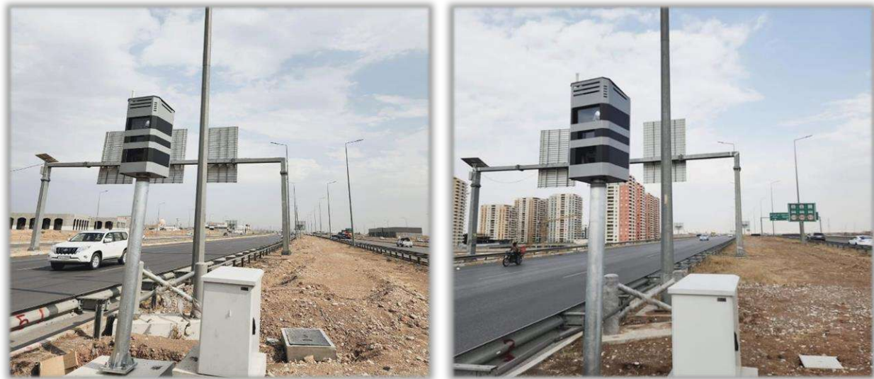
Fig 11,12 P2P cameras in Erbil-120m Street
