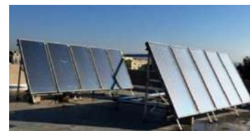
Figure 1. Flat plate solar collectors' arrangement
