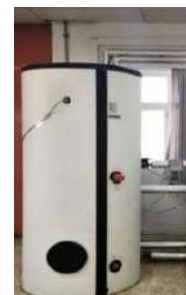
Figure 2. Water storage tank
