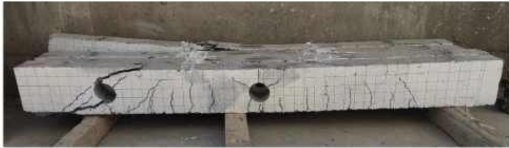
d) The patterns of crack observed and the failure mode for specimen SBLSF.
