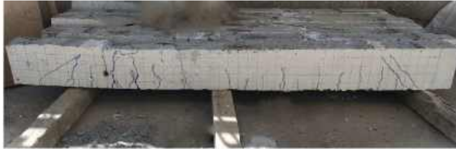
a) The patterns of crack observed and the failure mode for specimen DCB.
