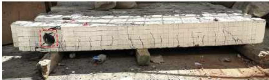
d) The patterns of crack observed and the failure mode for specimen DBLSS10.
