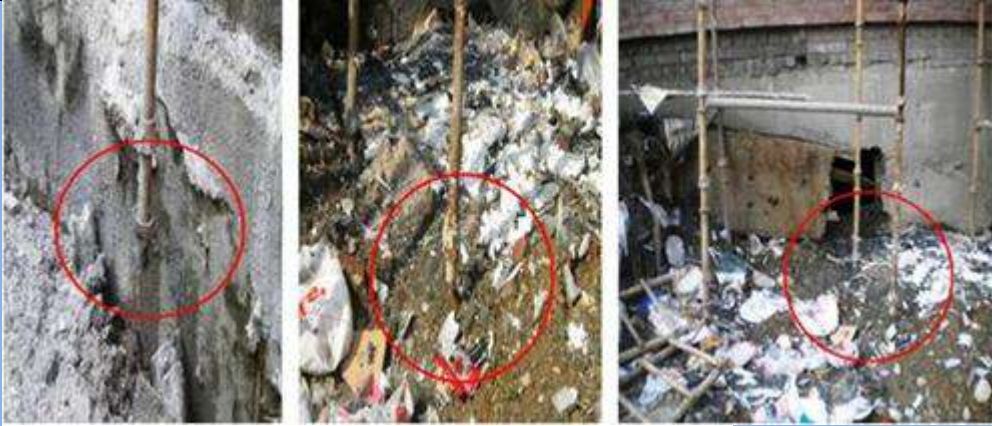
Fig.: Scaffolding Provided Without Foot bearing Plates
